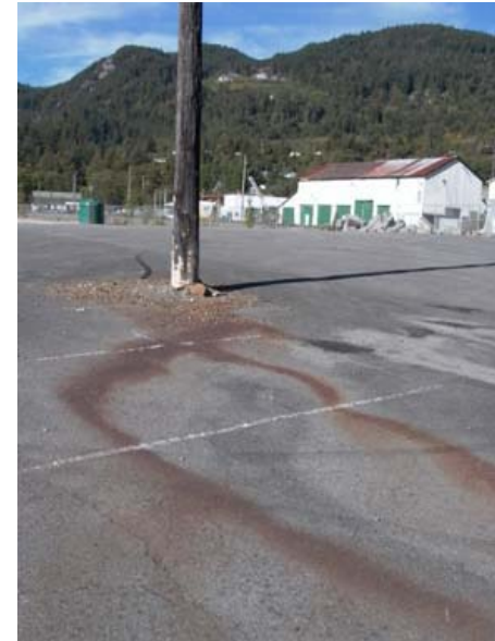
Leaching of metal rich sediments. Beach front parking lot, Britannia Beach, September 2003.
