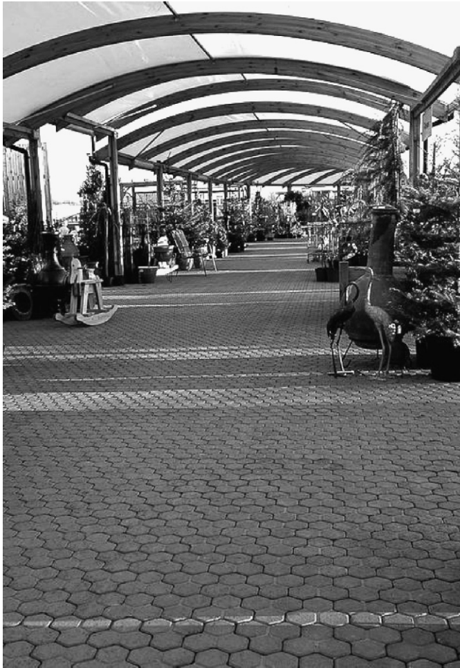
Fig. 1. Modern permeable pavement tanked system example with water recycling facility at Sanders Garden World (near Bristol, England, UK); picture taken by Mr. P. Smith in 2001.
